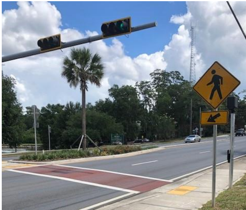
Figure 5.2-8. Midblock Traffic Control Signal
