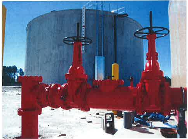
Industrial Water Supply Facility, Suwannee County
