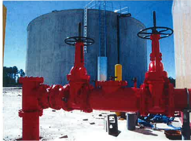
Industrial Water Supply Facility, Suwannee County
