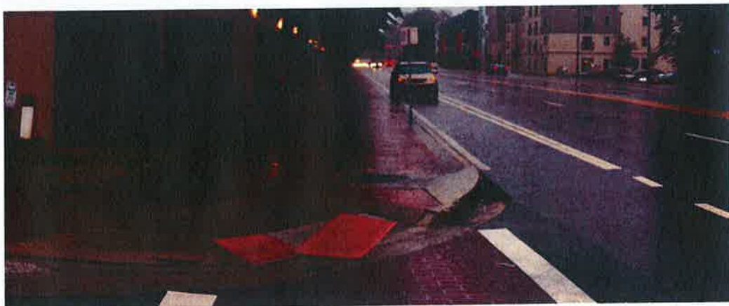
And uneven sidewalk/debris
